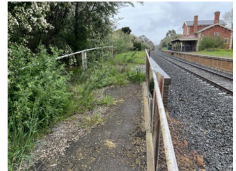
View of the existing eastern platform (on left) with environmental weed overgrowth damaging heritage infrastructure behind it.
