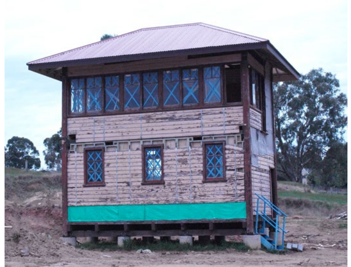
The Lions' new clubhouse in the refurbished Signal Box A from the Bendigo station has new windows and roof.
